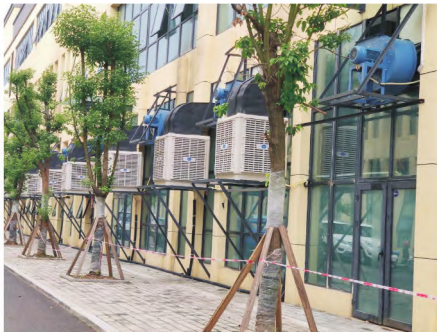
图 1 蒸发冷却空调在生产车间的应用 Fig.1 Application of evaporative cooling air conditioning in production workshop
